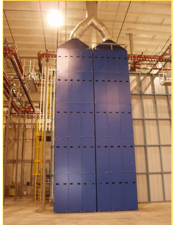
Gas fired catalytic infrared minimizes contamination in the powder curing oven.
